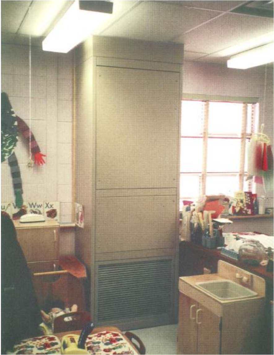
WALTHAM SOUTH ELEMENTARY SCHOOL – UNIT VENTILATORS
